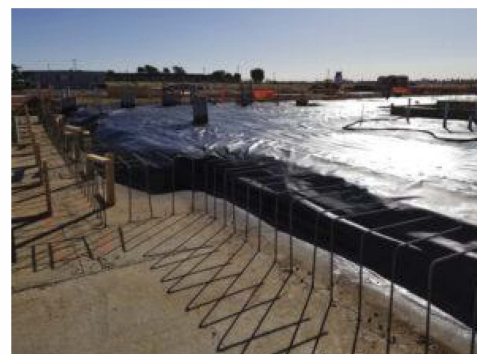
Vapor intrusion mitigation system (i.e., vapor barrier) installation during building construction at aerospace facility. (photo courtesy SCS Engineers)
