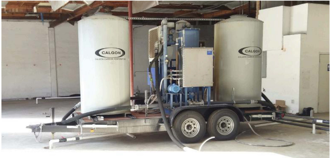
Soil vapor extraction equipment in former industrial dry cleaner. (photo courtesy SCS Engineers)
