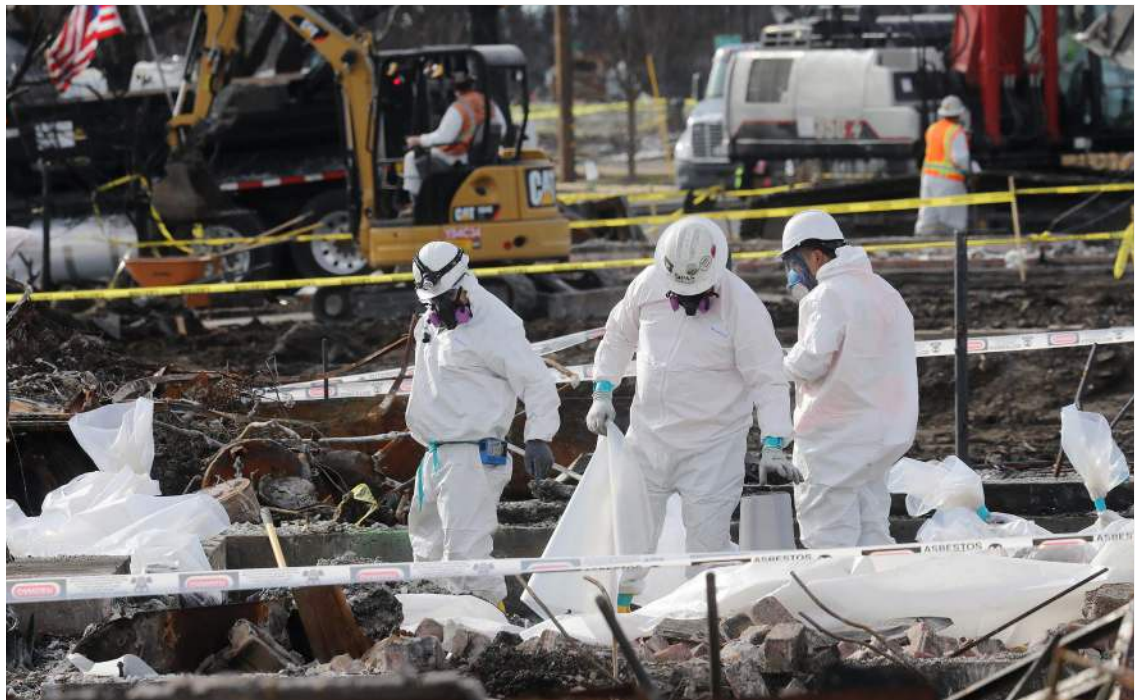
Workers remove asbestos-laden debris exposed by the Tubbs Fire in Santa Rosa, Calif. | The New York Times
