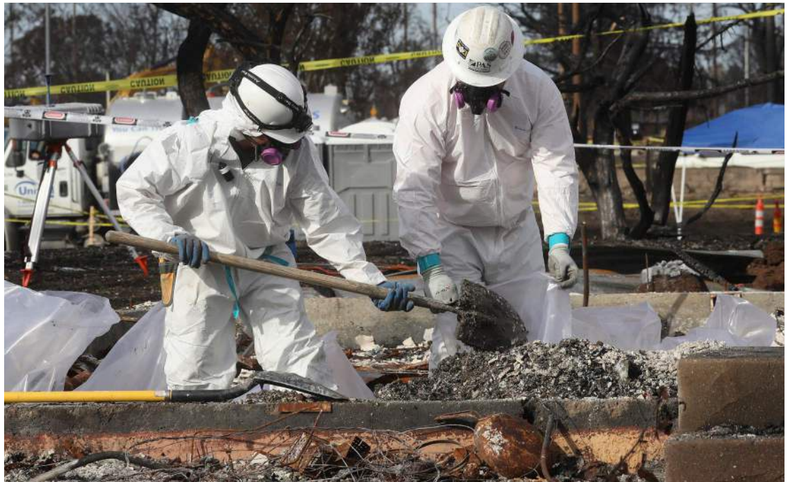
Workers clean up debris contaminated with asbestos in a burned home in Coffey Park, Calif. | The New York Times
