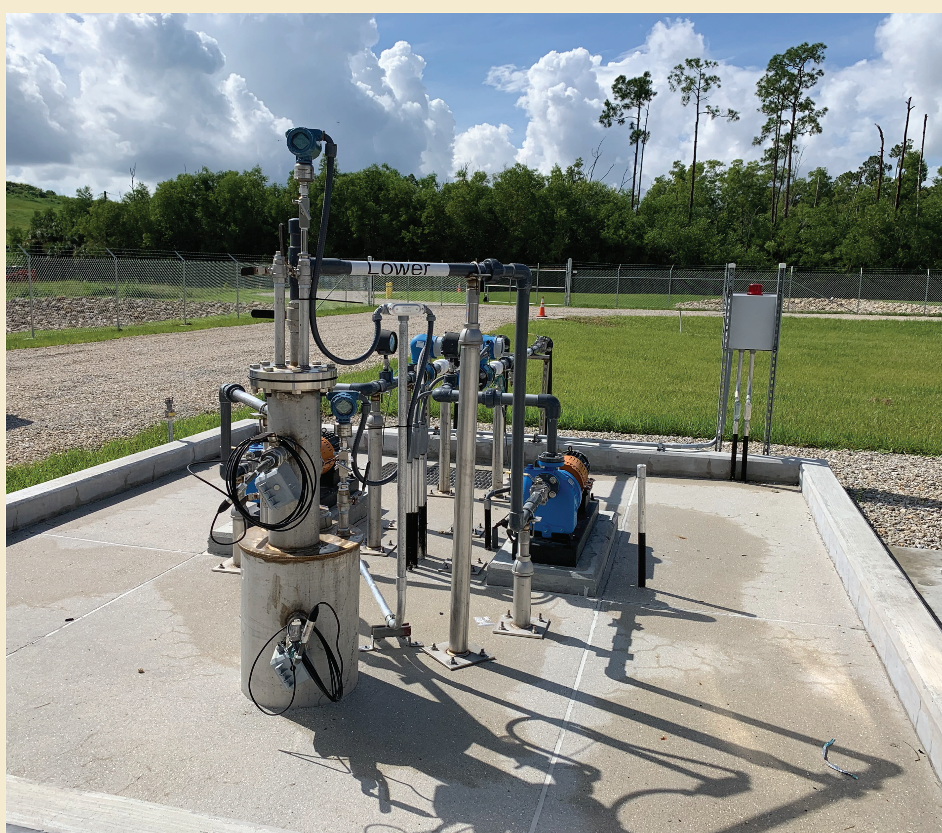
Dual Zone Monitoring Well
