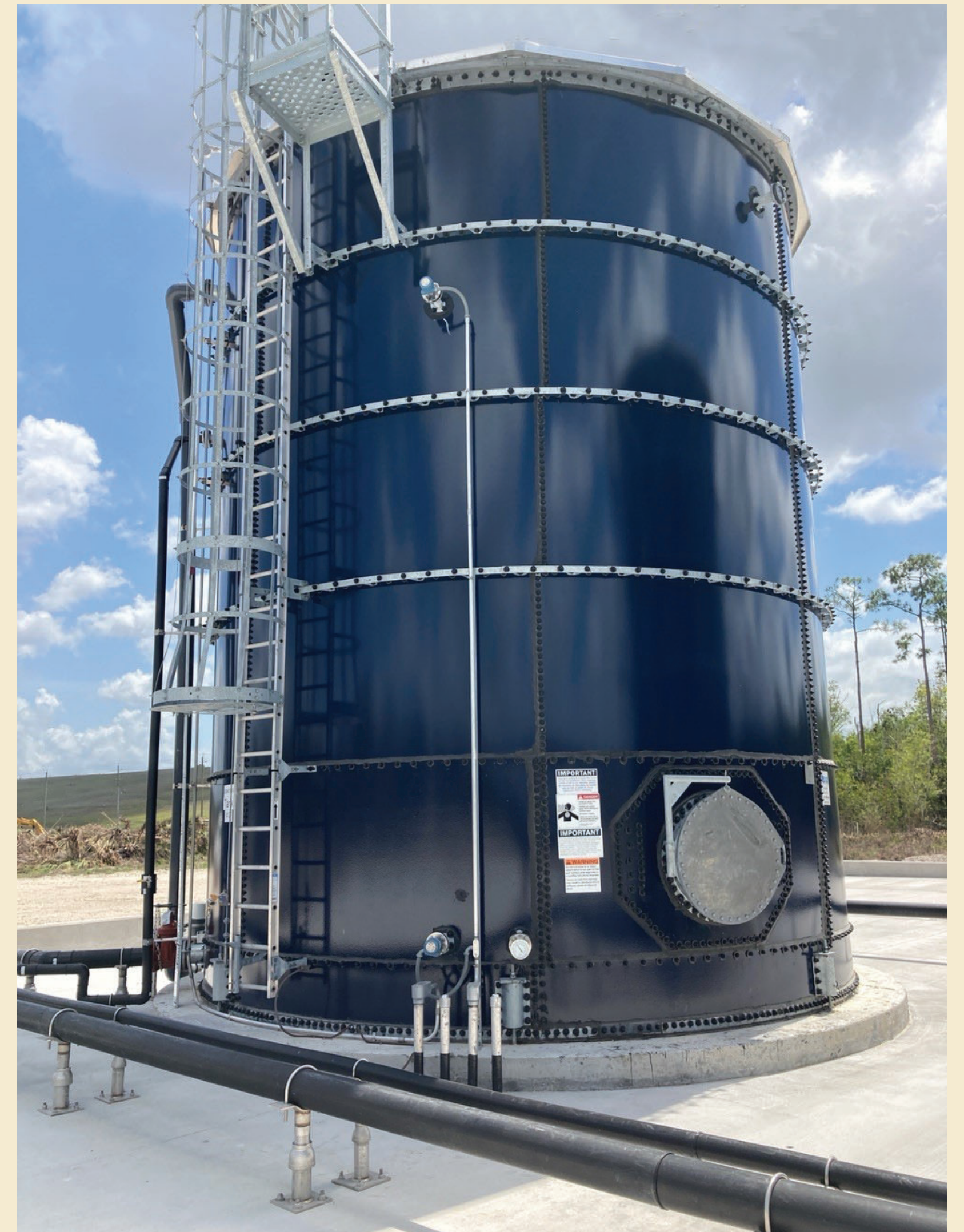
Aboveground Storage Tank
