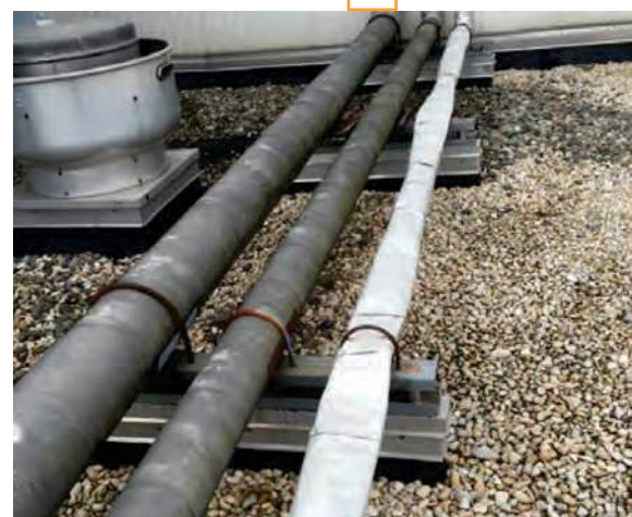
Insulation breakdown, maybe after an army stepped on the pipe
