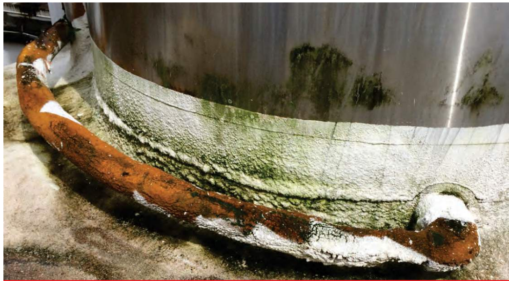
Armaflex insulation, mastic coating, and multiple layers of mold.
