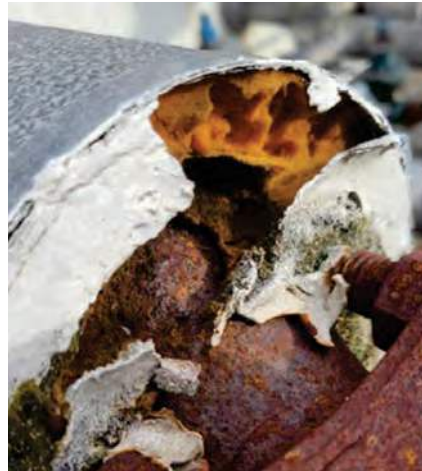
Deteriorated mastic coating at the end of insulation
