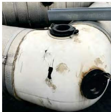
Deteriorated PVC elbow, but, by gosh, we've inspected it.
