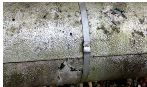
Protective jacket deterioration.
