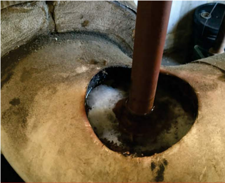
Had to add a pipe but ran out of money to repair the insulation.
