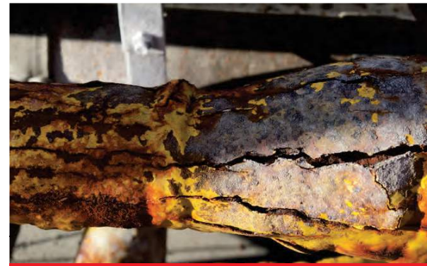
Extreme corrosion on a condenser drain line.
