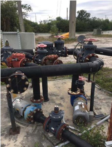
Booster pumps on a network of leachate force mains before connection to an offsite discharge line
