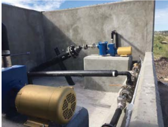
Pumps on the primary and secondary risers at a disposal cell leachate structure
