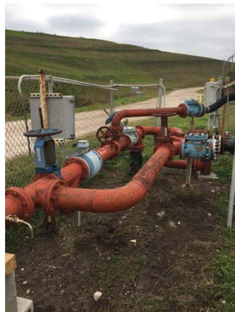
A junction of leachate force mains coming together from various operations
